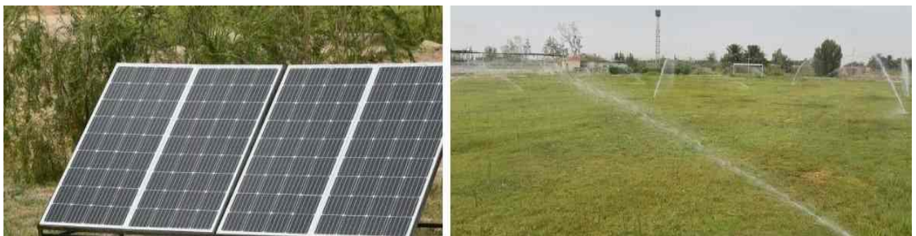
Spray watering using solar power
