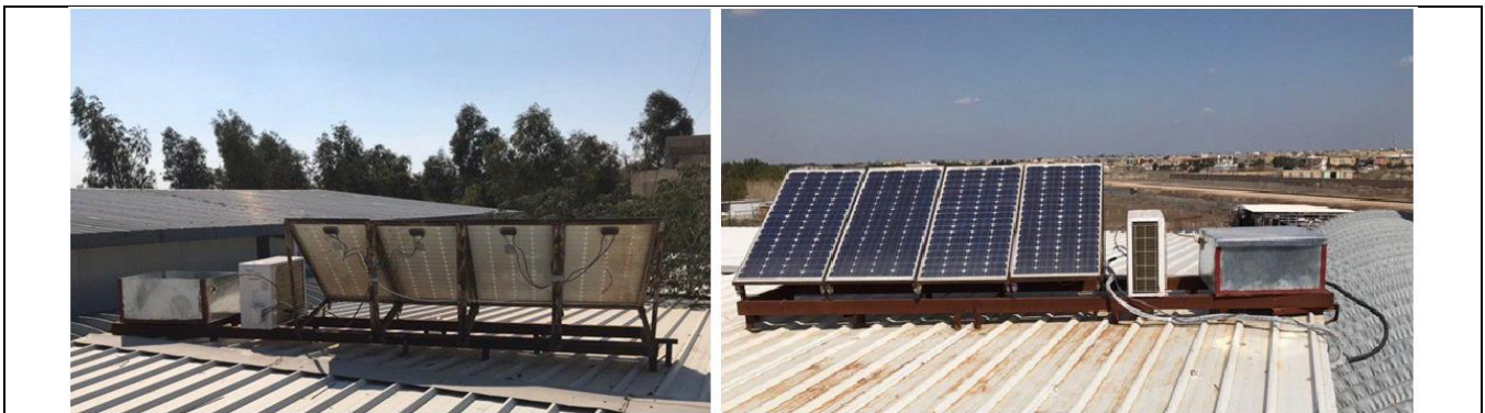
Air conditioning using solar power
